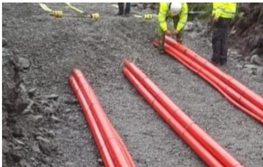
Plate 4-8 Typical Trefoil Cable Trench View
